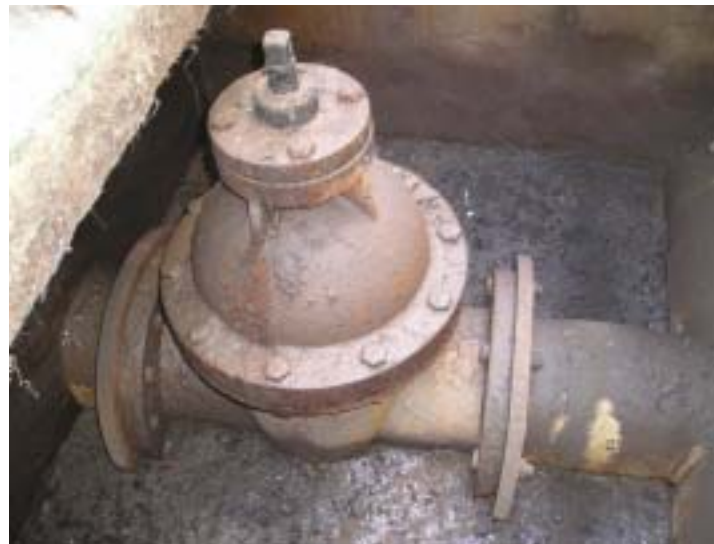
Figure 7.3 Marcala Sludge Valve
