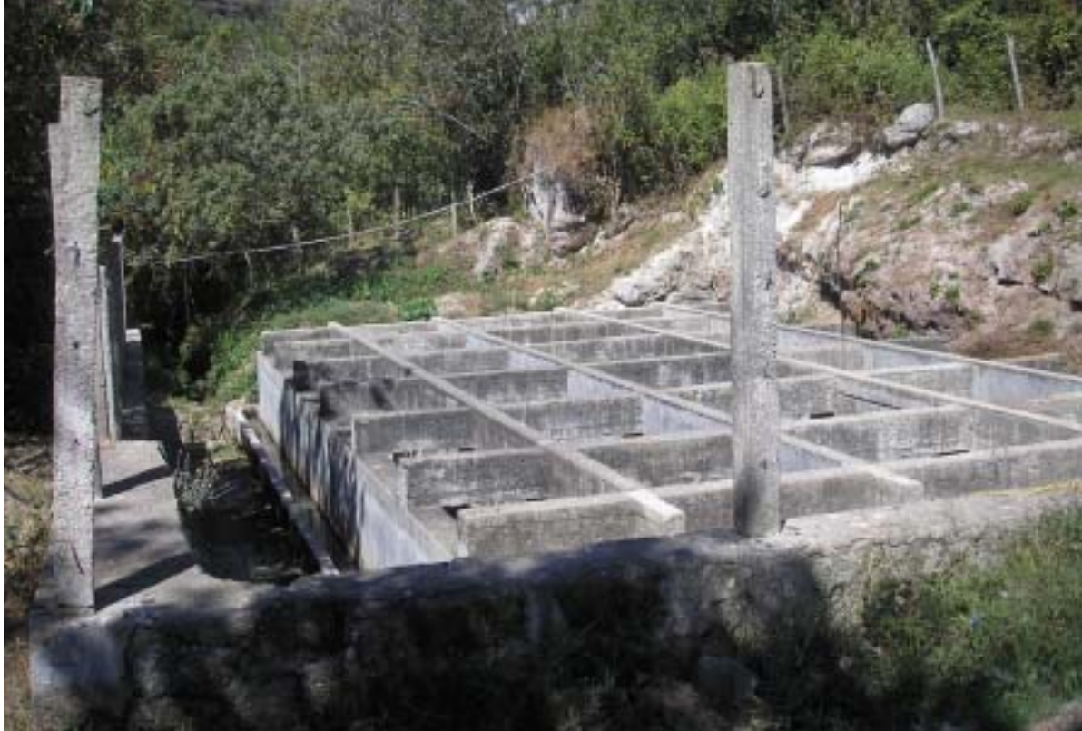
Figure 7.1 Marcala Imhoff Tank
