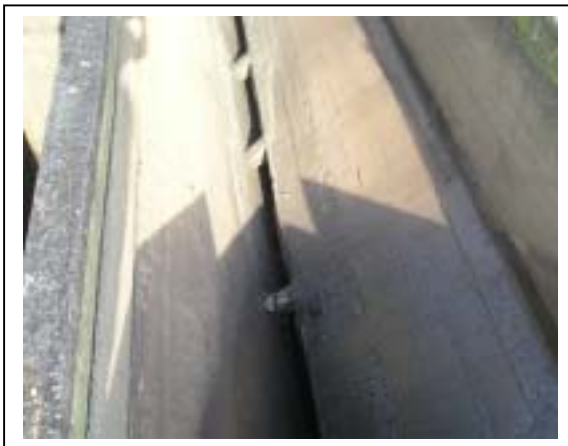
Figure 5.5 Inside View of Sedimentation Chamber
